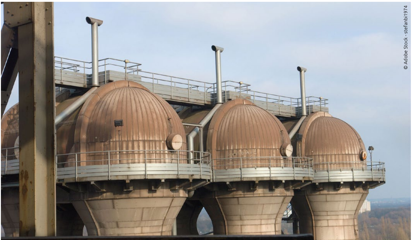
Fig. 1 Pyrometers measure the temperature of the grating refractory bricks in the stove dome from the cupola
