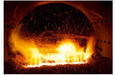
Installation de combustion
